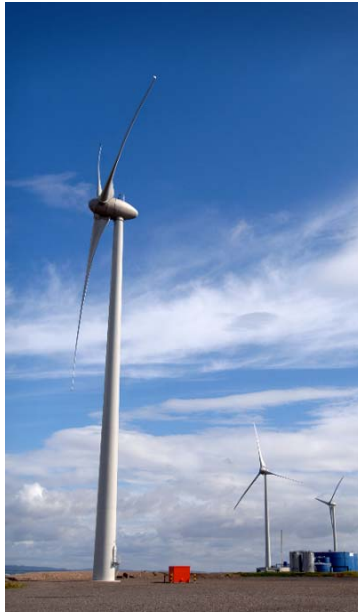
Figure 26, 2 MW Enercon wind turbine cluster at Bristol Port
