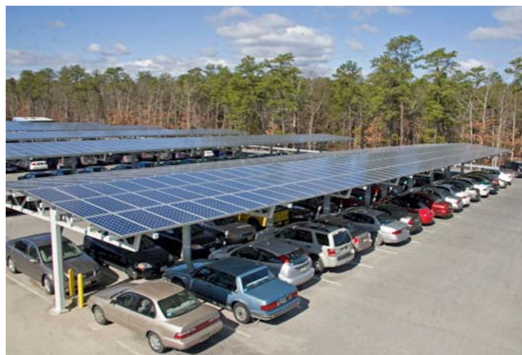
Figure 31, Solar PV array over parking area The Richard Stockton College of New Jersey parking array
